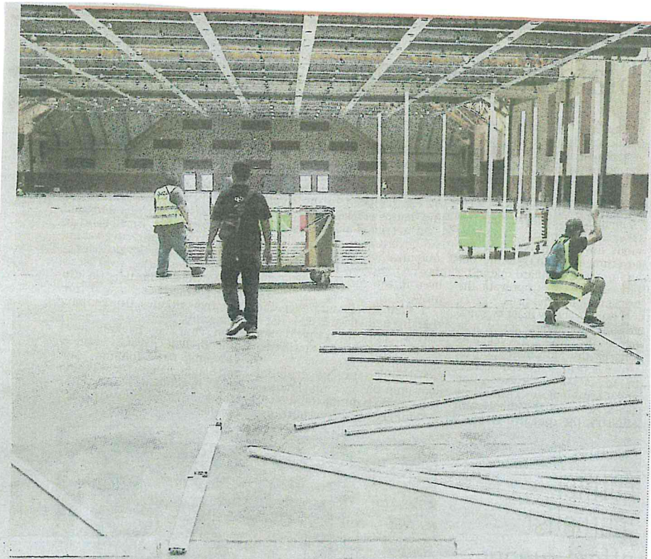
The Malaysia Agro Exposition Park Serdang in Selangor is being converted into a makeshift hospital. PIC BY MOHD FAULI HAMZAH
